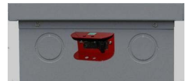
Battery box with 250 amp DC breaker and optional protector. Remove entire knockout.
